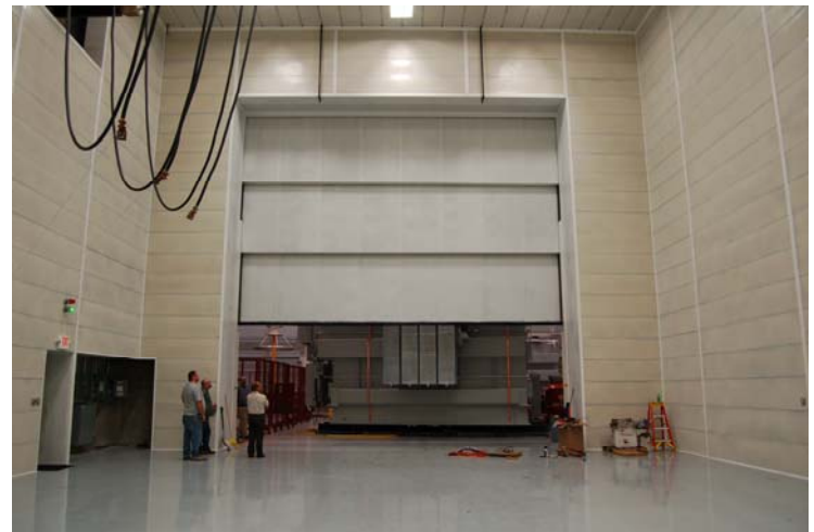
Waukesha Electric Transformer Test Facility Constructed by Noise Barriers LLC in 2007
